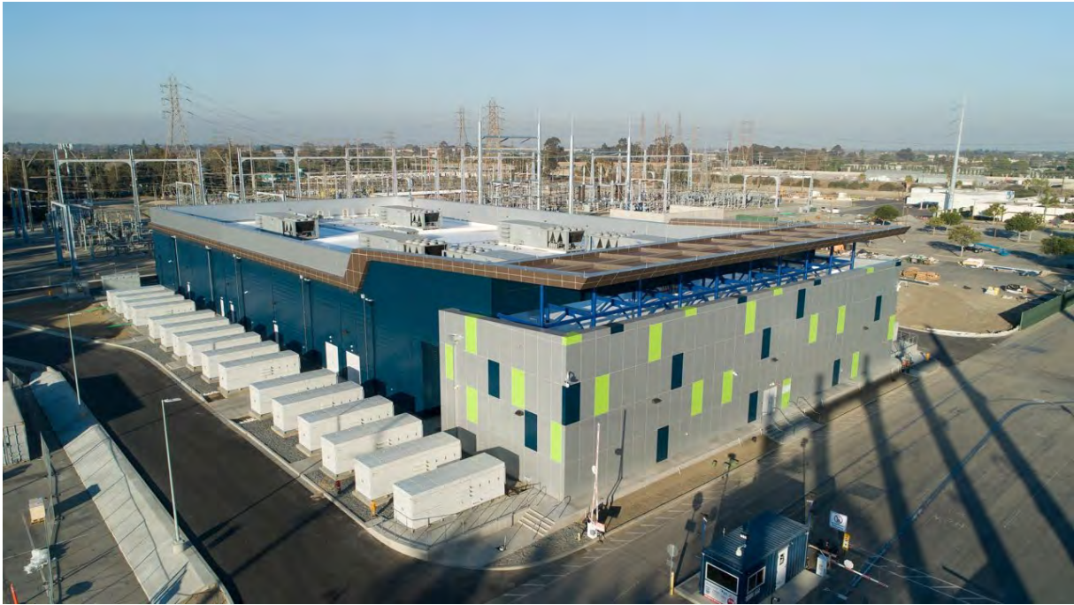
Figure 2: Los Alamitos 100MW / 400MWh BESS (Capacity Reserve and Energy provider)
