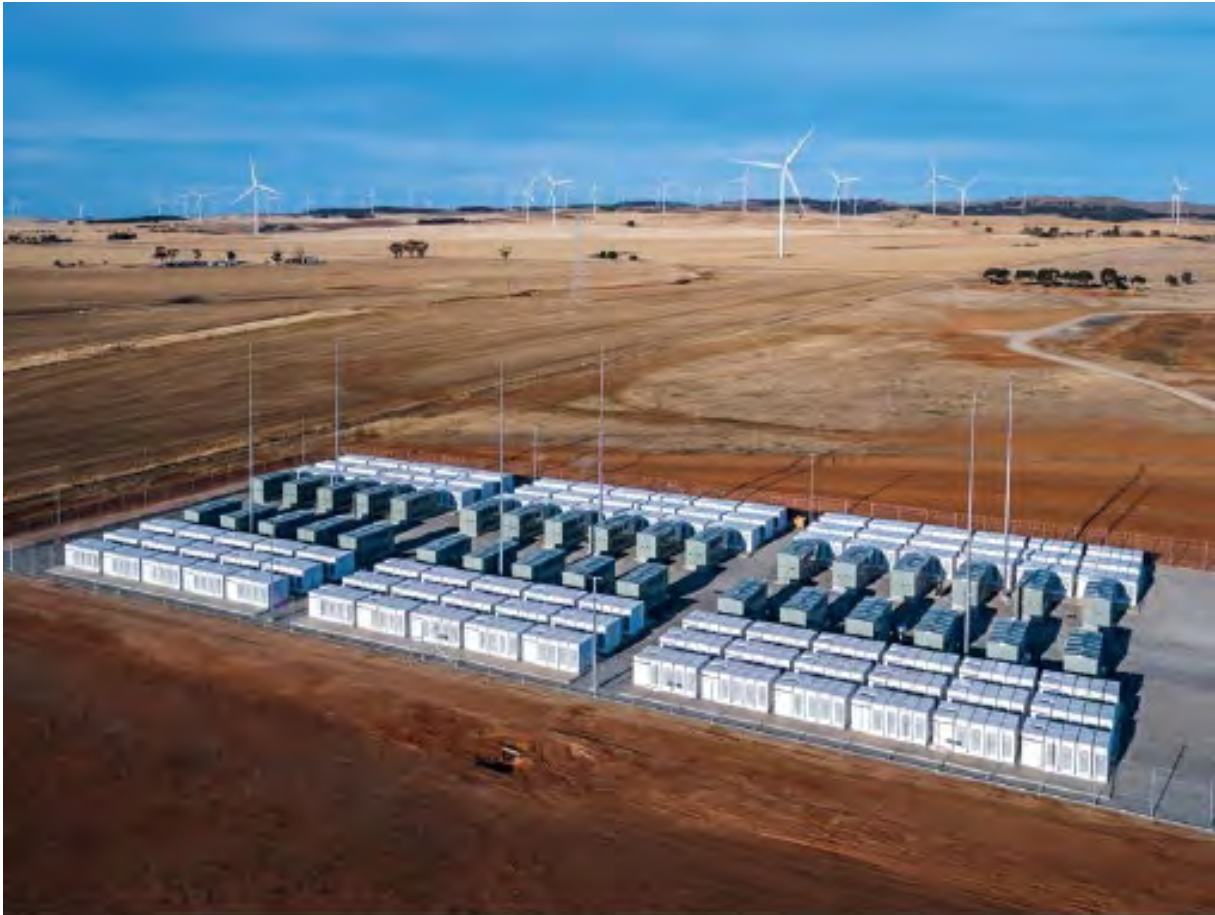
Figure 1: Hornsdale 100MW / 129 MWh BESS (Fast Acting Stabilizer & Energy provider)
